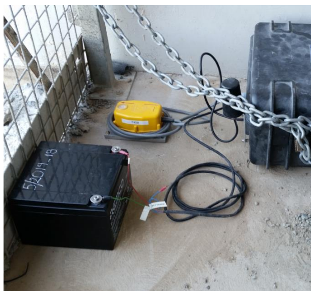
Figure 2 – Vibration Monitor Placement at R2
